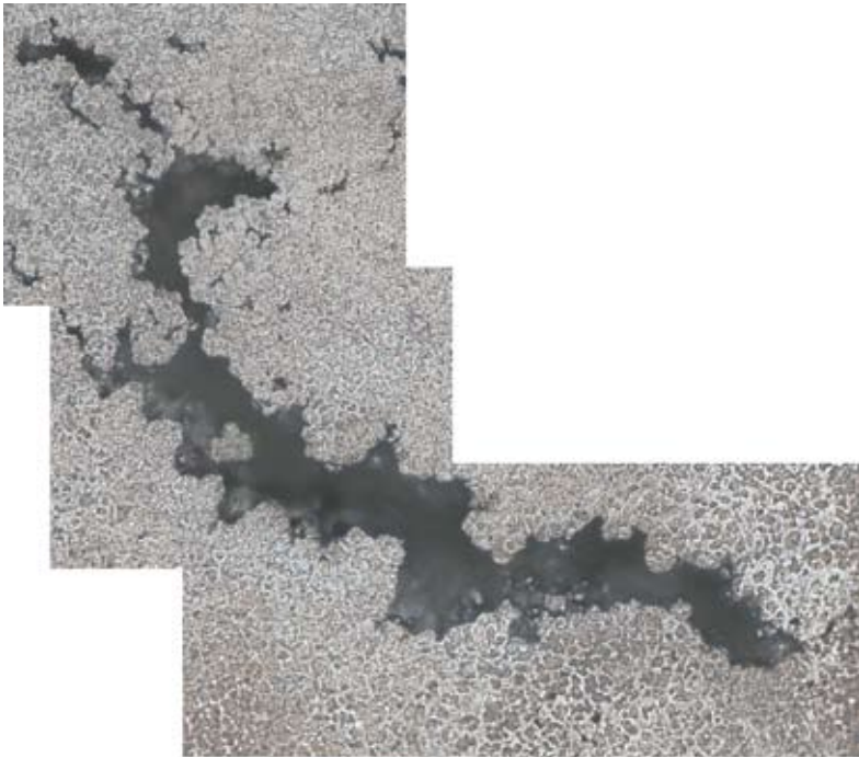
Panorama: a crack is followed beyond the image field. Only the required images are acquired.
